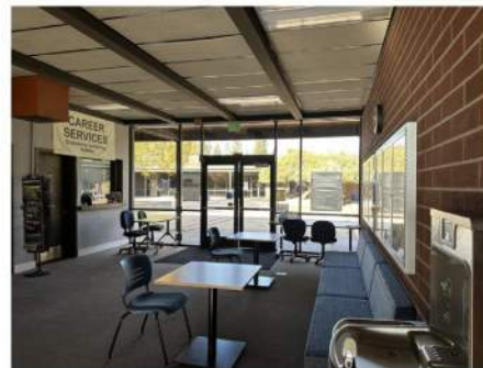
EXISTING SUSPENDED CEILING SYSTEMS REDUCE PERCEIVED HEIGHT, HIDE BEAUTIFUL STRUCTURE & DO NOT TAKE ADVANTAGE OF REFLECTED LIGHT OPPORTUNITIES
