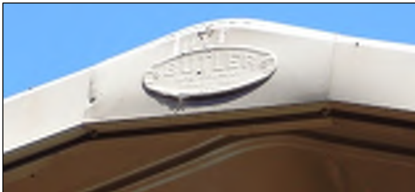
Figure 3: Storage Building roof peak, south faced, detail of manufacturer's faceplate, view north.
