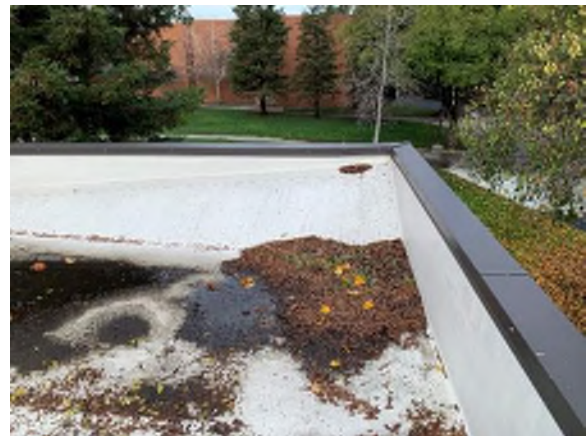
Photo 22: Debris on North Building roof.
